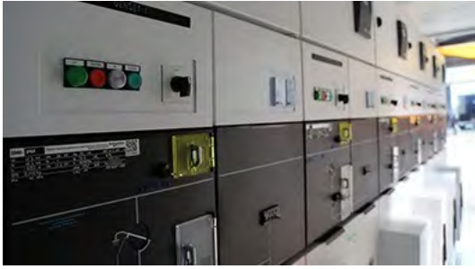
Medium voltage switchgear
